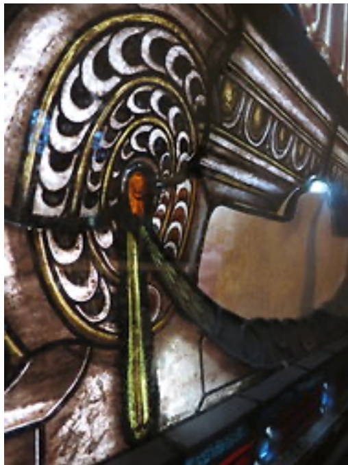
Another window at St. Mark's shows the kind of damage that was repaired on the Stuyvesant memorial: buckling and loss of glass. David W. Dunlap/The New York Times
